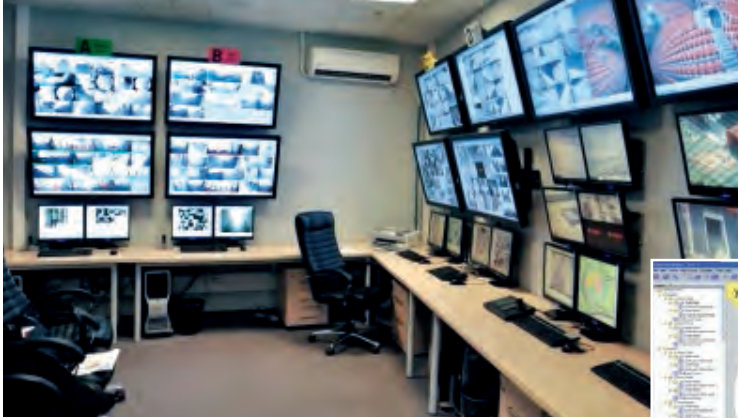
Control center with MxCC workstations and 42" live image monitors
